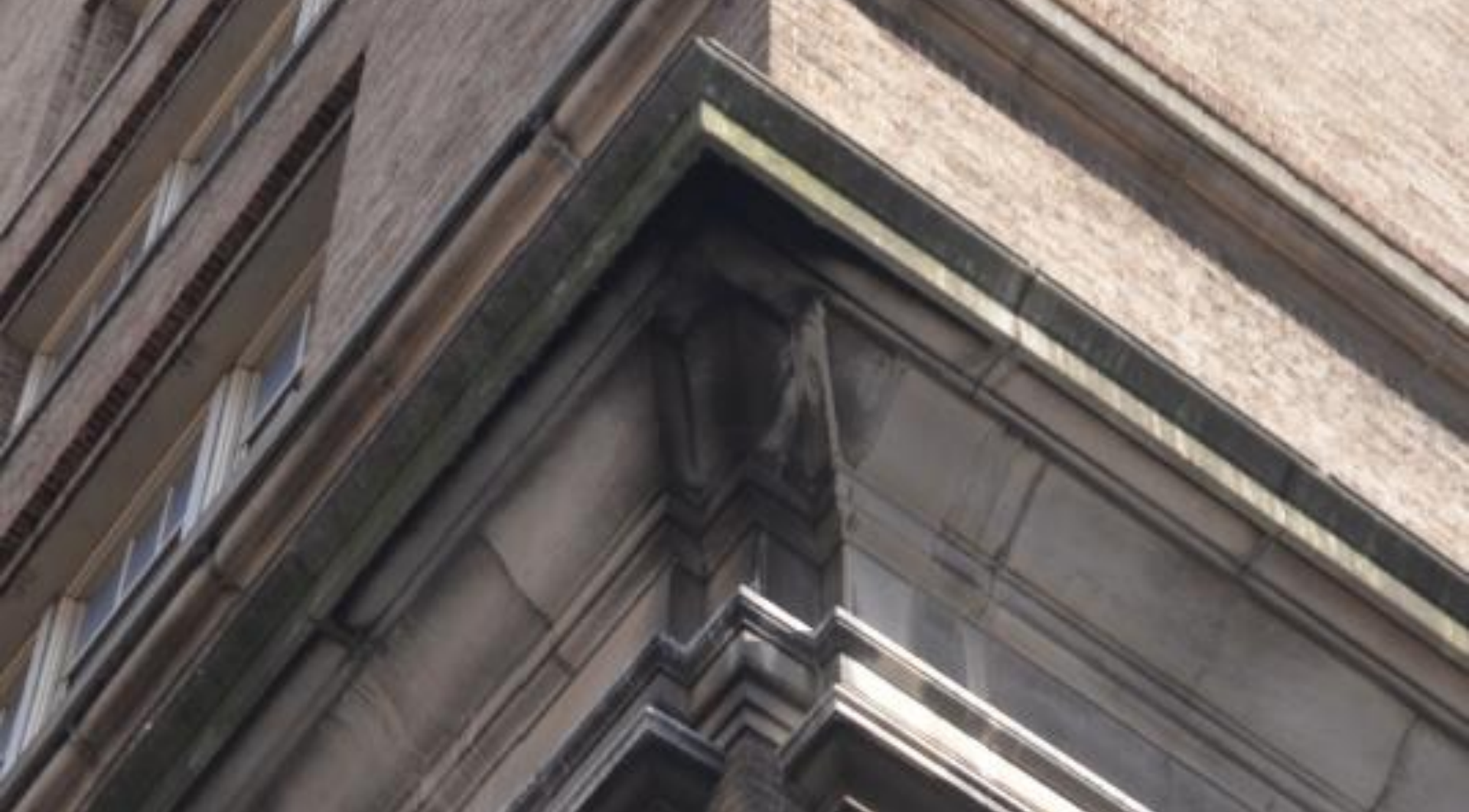
Photo 385: Cornice above the 2 nd floor at the Northwest corner of Original Building
