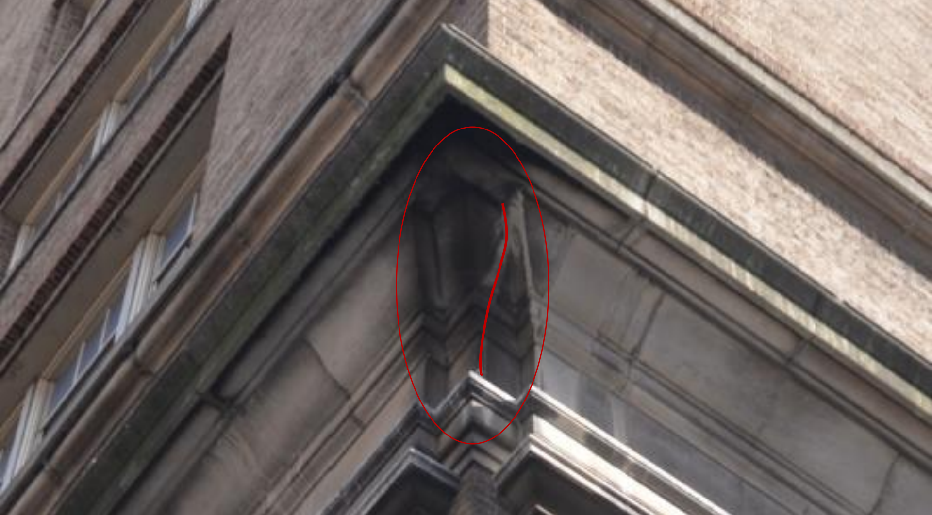
Photo 385: Cornice above the 2 nd floor at the Northwest corner of Original Building
