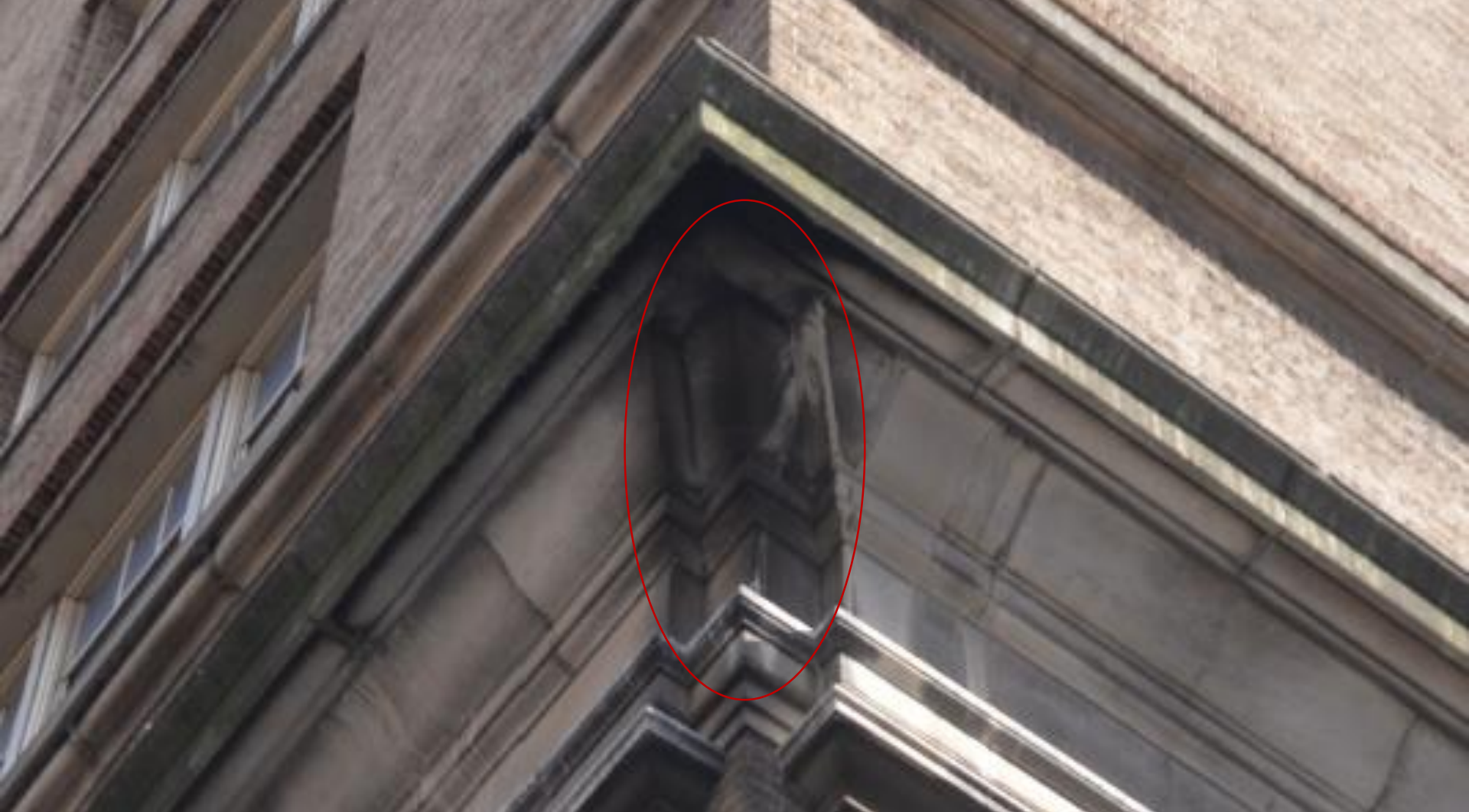
Photo 385: Cornice above the 2 nd floor at the Northwest corner of Original Building
