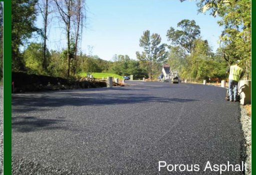
Stone infiltration bed
