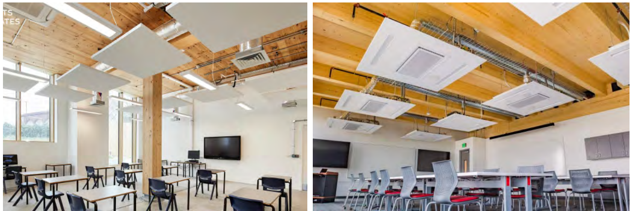
Figure 39. Ceiling Clouds by Overcast Innovations at UWMilgard Hall, Seattle, WA (left, clouds separate from MEP devices) and Catalyst (right, MEP devices integrated into clouds), Spokane, WA
