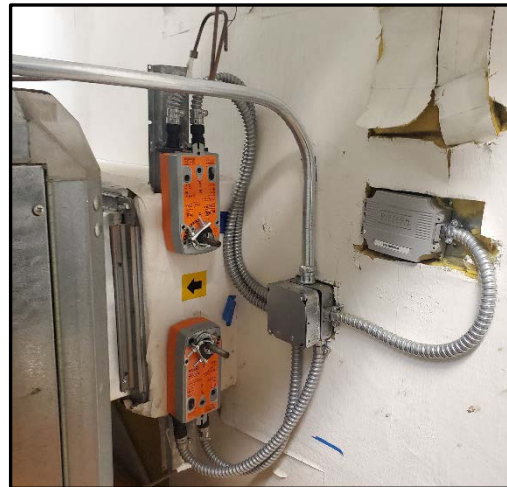
Photo 4: AHU-1 Modulating OA Dampers
