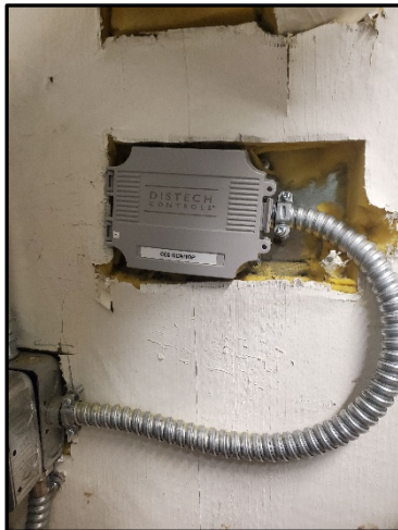
Photo 3: AHU-1 CO 2 Monitor
