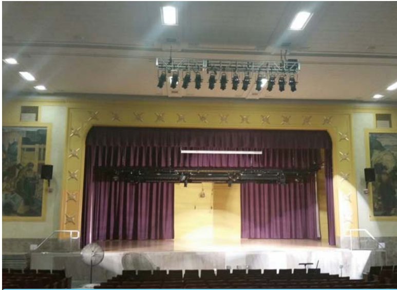
PS 113 Bronx - Auditorium Upgrade
